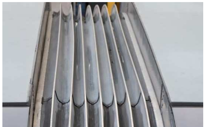
IMAGE 2: Likewise cleaned just by rain: flexible corridor connection
